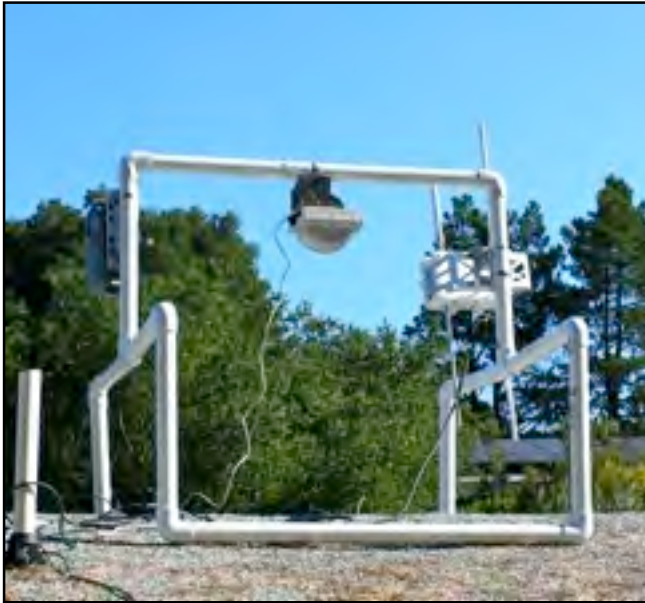
Fig. 2: Roof mounted APs, POE cable carries power only
